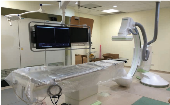
Figure 4 Interventional Nephrology Suite 2 (INS 2) was set up in 2015. It is equipped with fluoroscopy equipment for the performance of endovascular interventions.
